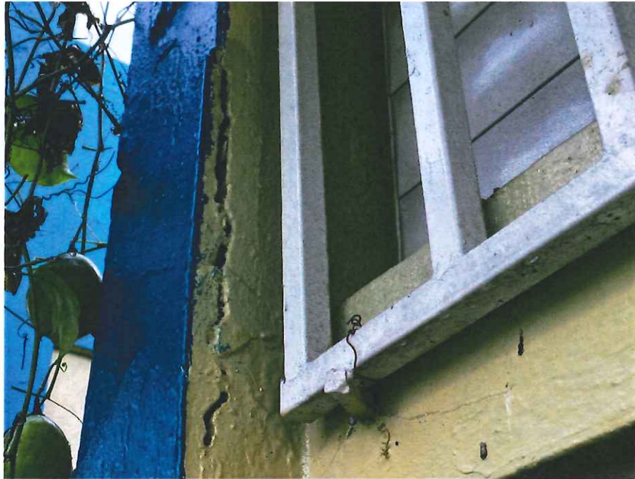
Photo 3: Crack at exterior column
