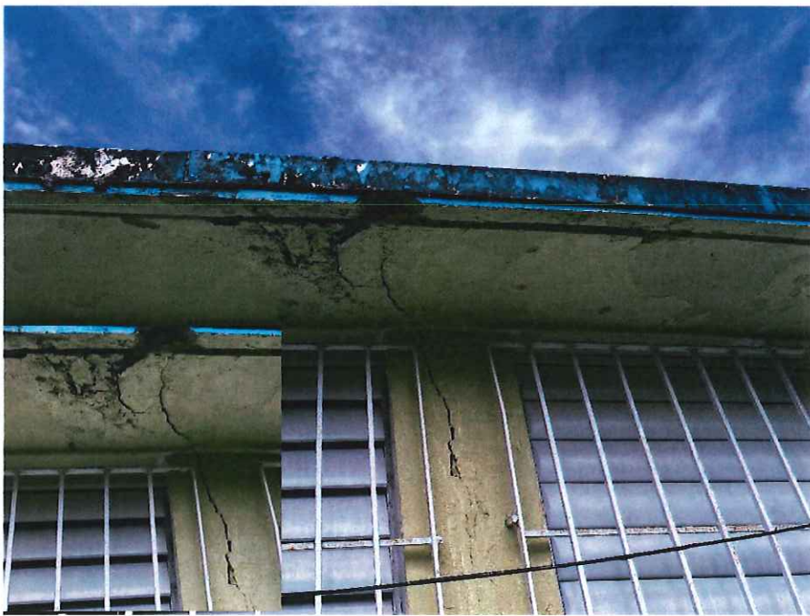
Photo 2: Exterior crack on column/eave intersection
