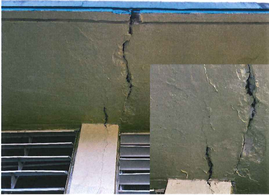
Photo 1: Exterior crack on column/eave intersection
