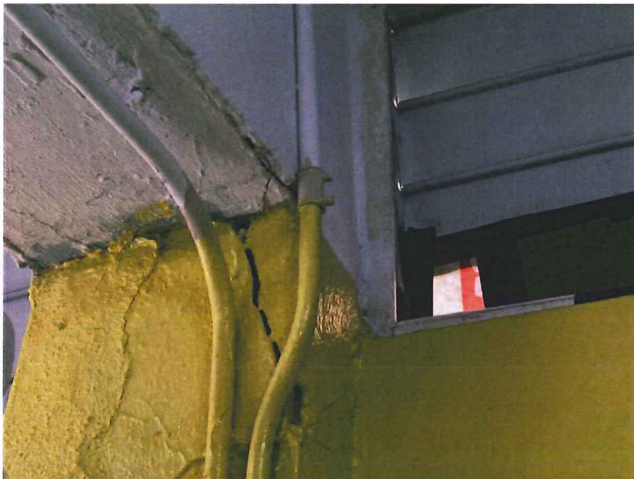
Photo 4: Crack on beam/column intersection
